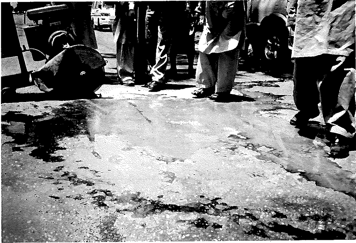
Photo No. 9 APPEARANCE OF CLAYEY - SILTY SLURRY DURING CUTTING OF 2' X 2' PIT RD No. 1885+385 Section 6 (N.B)
