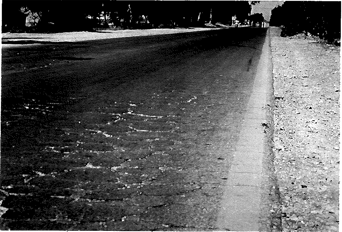
Photo No. 1 CRACKS VISIBLE ON PAVEMENT SURFACE (Rehabilitated Section)
